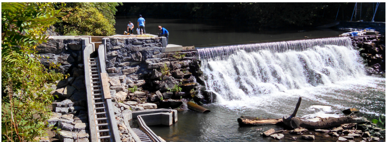
Fish ladder installed by the New York City Department of Parks and Recreation at the 182nd Street dam in the Bronx River.
